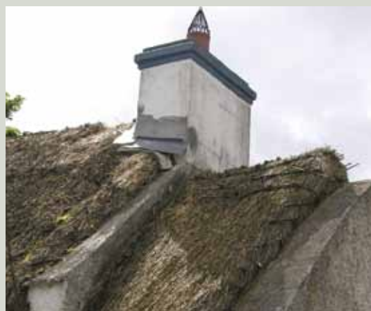
The poor quality flashing detail at the foot of this chimney stack is causing localised deterioration of the thatch
