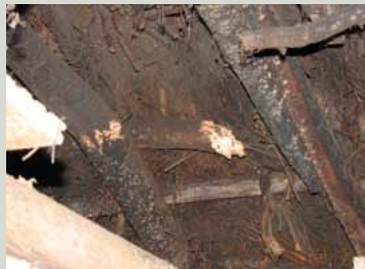
Broken roof timbers in a thatched house with evidence of furniture beetle infestation
