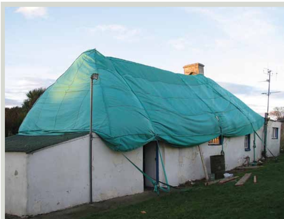
Temporary protection provided by canvas sheeting may provide a short-term solution in an emergency but can accelerate the deterioration of the thatch by preventing it from drying out
