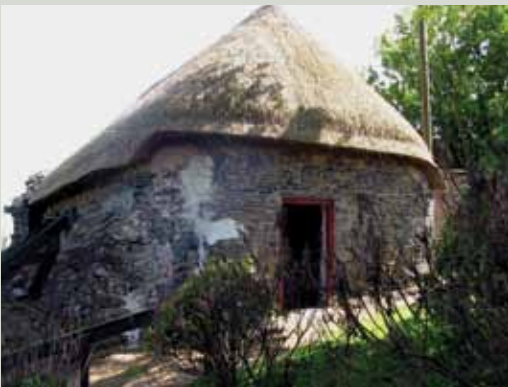
A single-cell thatched Mass house at Tomhaggard, County Wexford is believed to date from the eighteenth century and contain fabric of an even earlier building in its walls
