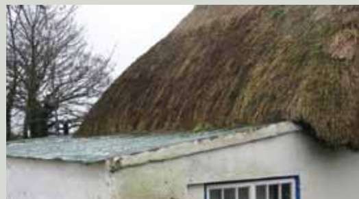
The end of the thatch sits on the lean-to metal roof of an extension. Rainwater shed from the thatch cannot drain properly and will eventually lead to rotting of the thatch
