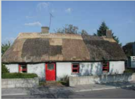
Regular patching and repair have always been features of maintaining a thatched building, a process which extends the life of a roof until such time as a full re-thatch is necessary
