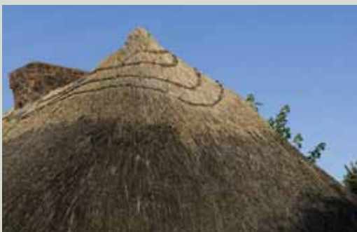
Rows of horizontal stretchers can provide a decorative detail in addition to their functional role of securing the ridge and other vulnerable parts of the roof, County Limerick
