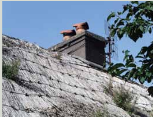
Now in poor condition, this example of a straw, pegged thatched roof in County Sligo is an increasingly rare survival
