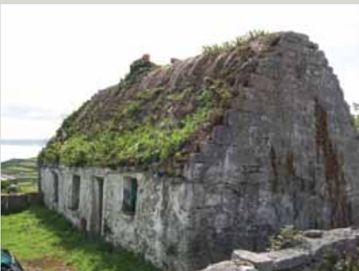
The results of lack of maintenance. Due to the fragile organic nature of the materials used in thatch, buildings can deteriorate rapidly when neglected
