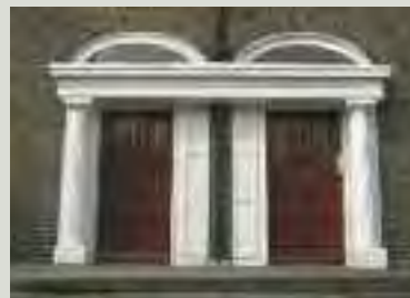
The inaccurately-detailed alteration of doorcases or other features will, in most cases, be to the detriment of the structure and often affect the character of an ACA also
