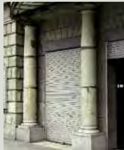
The entrance doors to this establishment have been fitted with roller shutters. Although the physical impact has been minimised, the closed shutters nonetheless have a large visual impact on the appearance of the structure and the streetscape. This impact can sometimes be overcome with the use of internal demountable grilles, a less visually obtrusive option of securing a historic shopfront, especially when painted a dark or neutral colour
