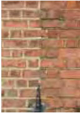
Repointing which uses methods and materials other than the originals may alter the character of the building as has happened with the example on the left of this photograph
