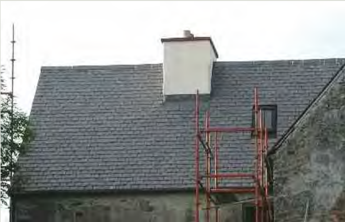
Valentia slate, famed for its qualities during the nineteenth century and again being quarried on a commercial basis, is here used on a conservation project. The use of regional slate types can be an important aspect of local distinctiveness and research indicates that slate native to a region generally performs best in the climatic conditions of that area. When undertaking restoration works to important roofs, the feasibility of reopening a local quarry to supply new slate should be investigated
