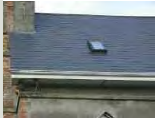
Inappropriate alterations to roof shapes and details detract from the character of a structure; in this case the new roof has overhanging eaves with uPVC fascias, soffits and rainwater goods - an incorrect design using inappropriate materials on this former Board of First Fruits church
