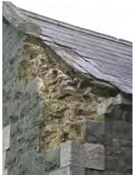
Urgent works may be needed to secure the fabric of a building following damage
