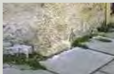
The injection of a damp-proof course may result in visually obtrusive pockmarks on the external walls of the building and is unlikely to be fully effective in rubble walling
