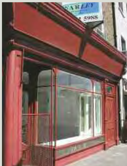
The essence of good repair work is to retain the maximum amount of viable fabric that contributes to the character of the shopfront, to carry out the work using proven methods of repair and to fit appropriately detailed new elements where necessary. This shopfront was carefully repaired with grant assistance from the local authority
