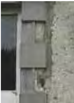
Poorly-executed and badly-located service installations can have a serious effect on the character and appearance of a protected structure
