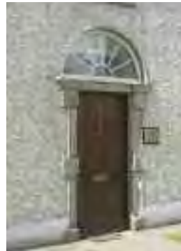
The replacement of original features, in this case the fanlight and door, with substitutes made from inappropriate materials should not be considered exempt
