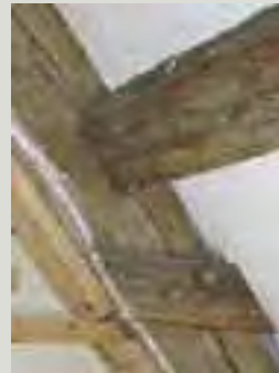
The structural components of a roof may contribute to its character. Here a seventeenth-century pegged oak roof structure survives largely intact, with the carpenter's numbers visible on some timbers
