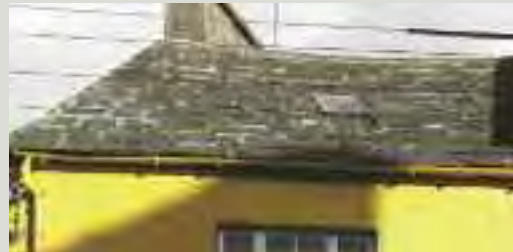
Moher 'slates', a regional type of roof cladding once common in Co. Clare, are in fact thin slabs of limestone dressed as slates. Stone 'slates' are rare survivors and, wherever possible, should be maintained in place with minimum intervention
