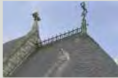
Ridge tiles, finials, iron cresting and weathervanes are found on many structures and give a building its distinctive outline against the sky. Repairs should follow best practice for each particular material
