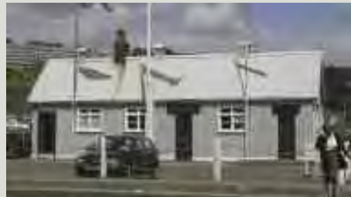
Corrugated iron sheeting may degrade through cracking or rusting (caused for example by sea spray in maritime areas) to a point where replacement is necessary. This recently-reclad harbour-master's office has replaced the original, but rusting, corrugated iron with a modern profiled metal sheeting
