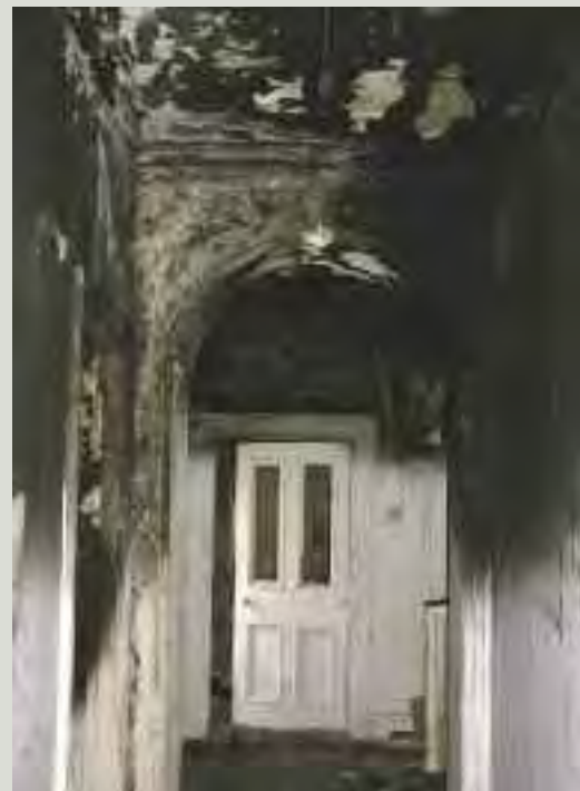
The true extent of damage to important interiors may be disguised by smoke-blackening and blistered paint. Careful spot cleaning of the stained and blistered surfaces and examination of lath and plaster linings will be needed to establish whether or not decorative interior plasterwork or joinery is capable of repair
