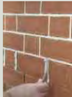
Where the repointing of historic brickwork is proposed, the specification of the mortar and the style of work to be used in repointing should be provided. Where specialist work will be required such as wiggling and tucking, demonstrated here, the work should be undertaken by experienced personnel
