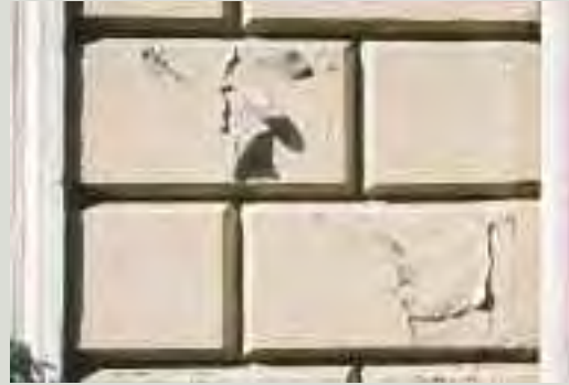
Applying impermeable paint to render or masonry can inhibit the necessary passage of moisture through the fabric. Unsuitable paints may peel off, sometimes shortly after application
