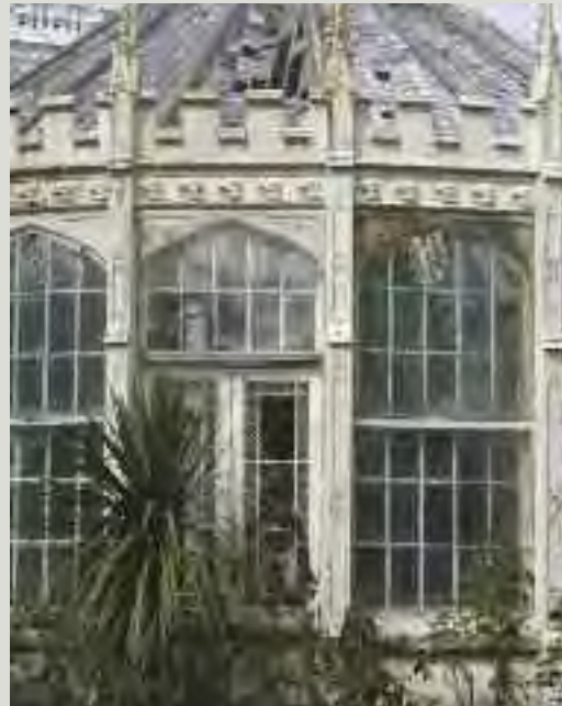
While it may sometimes be necessary to carefully dismantle an ironwork structure for repairs, some structures may consist of iron-clad sections on timber and masonry supports and may be more difficult to successfully dismantle and reassemble
