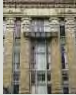
Terracotta, faïence and glazed ceramic tiles are all used to good visual effect in cladding or decorating the walls of buildings
