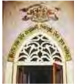
In these examples, interior features of importance have been damaged and any proposed repair will require to be carried out to a high standard in order for the work to be considered exempted development
