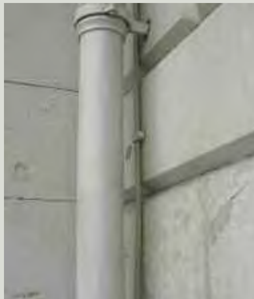
Lightning conductors may be a requirement on tall or otherwise vulnerable structures. The conductors should be channelled to earth unobtrusively; this example shows a discreetly coloured lightning conductor carefully concealed behind a downpipe
