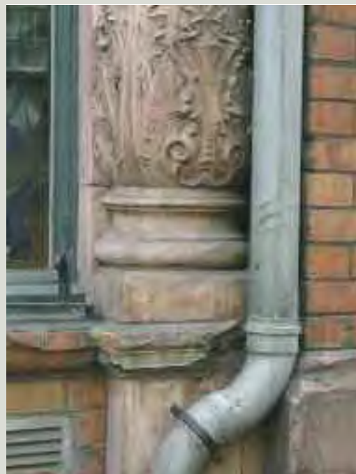
The ill-considered fixing of new items such as pipework to the principal elevations of structures can adversely affect their architectural quality and cause physical and irreversible damage, as has happened in this case where a fine architectural element has been cut through to facilitate the location of a new pipe
