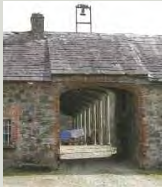
Undulations and previous repairs of good quality may all contribute to the character of a roof. Any necessary works should leave intact original detailing such as this raised archway roof, as it provides definition to the entrance bay
