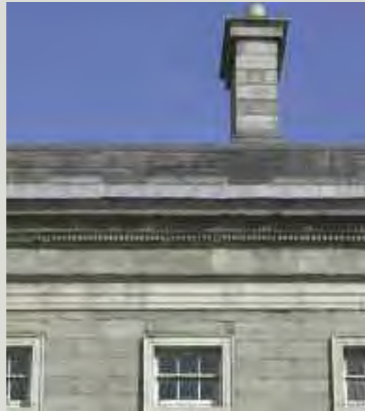
The eaves of a building can be vulnerable to weather-related problems, typically parapet walls become saturated as they are exposed on both sides to rain. Problems will also arise where the blockage of the gutter concealed behind a parapet may not be readily noticed. However, where they exist, parapet walls are usually an important architectural feature of the building
