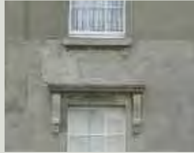
Localised re-rendering should be carefully specified to match the existing material. In this example, while the strength and texture may be adequate, the unmatched colouring of several patches is visually obtrusive
