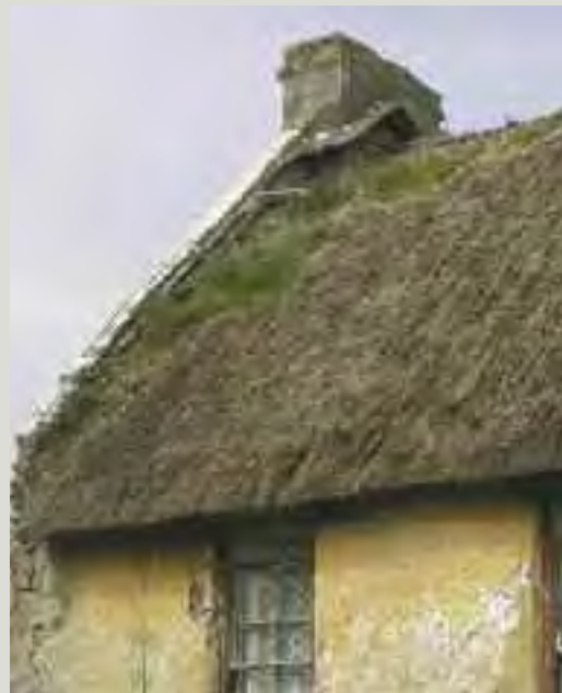
Thatched roofs can decay quickly once neglected. Therefore it is important to make their repair a priority if grant assistance is available and to ensure that a thatcher, experienced in methods traditional to the region, is employed
