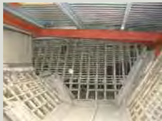
Old roof timbers should not be routinely stripped out as this can lead to a loss of character and the destruction of important historic elements. In this case, a roof structure, dated to the 1580s using dendrochronology, remains intact and, although no longer capable of taking the weight of cladding, is preserved beneath a new metal structure
