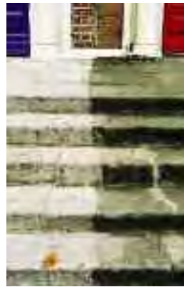
Uncoordinated programmes of stone cleaning can create aesthetic problems in terraces of similar buildings
