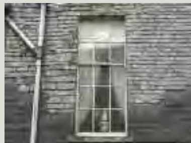
Slate-hanging should be carefully repaired where necessary using slates of a matching size and colour, with additions such as downpipes and vents carefully sited and fixed in order not to cause damage
