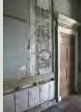
Later finishes or features may cover earlier elements of interest such as this sixteenth-century doorway, partly covered by re-used original panelling and an eighteenth-century doorcase; it may be necessary simply to record the earlier feature while retaining the high-quality later work in place undisturbed
