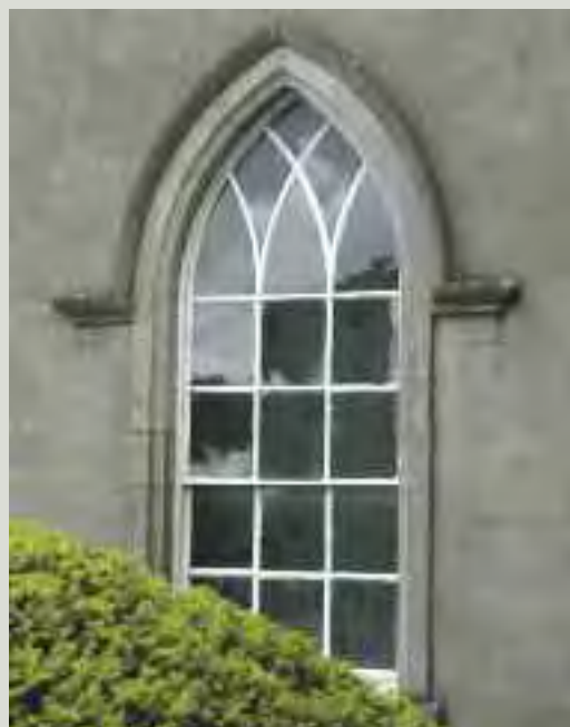
Fully-glazed blind windows such as this example are rare; they may be deliberately designed to ensure symmetrical fenestration (for example, where the plan form did not permit a window), or could represent later blocking of openings. It is commonly thought that openings were blocked to avoid paying window tax, which was in force between 1799 and 1851, however in Ireland there is little evidence to support this theory
