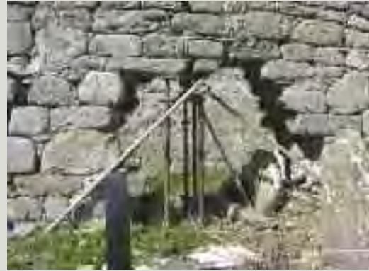
Structures may be in need of propping prior to, and during the course of, works which should be designed and installed to avoid causing damage to unstable fabric
