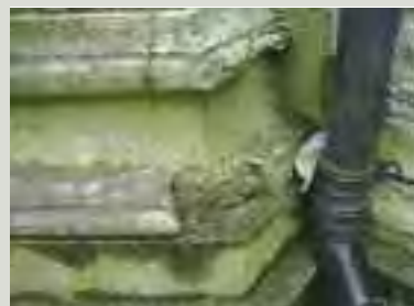
Damp problems arise more often from poor maintenance or poorly-executed repair works than from inadequate original detailing.
