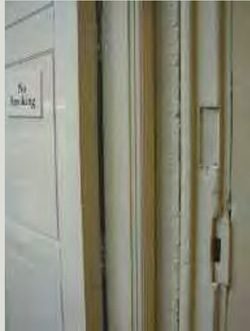
The reversal of a door to allow it to open in a different direction may require obtrusive alterations to a historic doorcase and may make the original hinges and locks redundant
