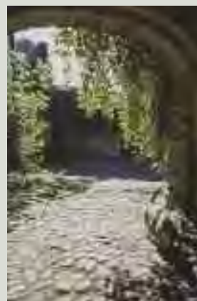
The wear caused by traffic over many generations across cobbles, setts, flagstones or brick pavements gives them a patina which often makes a significant contribution to the character of a protected structure or of an ACA
