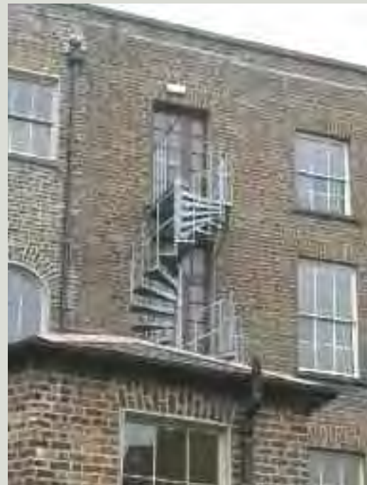
Proposals that require the conversion of original window openings into doors to facilitate escape will require very careful consideration and should avoid impacting on surviving early or original windows and on important elevations. There may also be a potential impact on nearby windows which may require re-glazing with fire resistant glass
