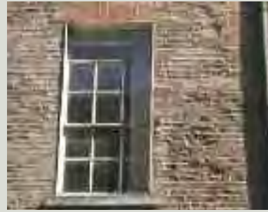
The decay of the soft handmade bricks of this façade has been accelerated by the use of extensive and poorly-executed cementitious mortar repairs coupled with strap pointing
