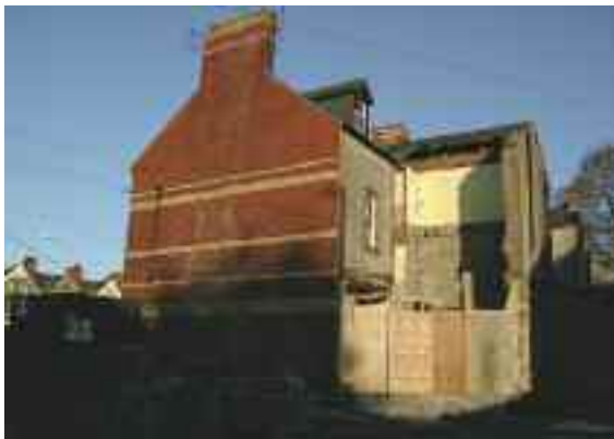
The demolition of a building's return can impact on neighbouring buildings also
