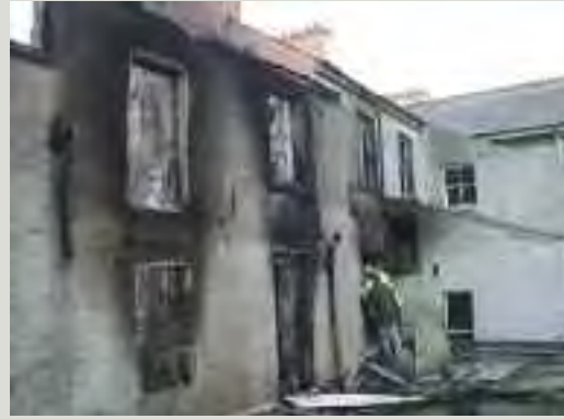
As soon as it is safe to do so, the surviving fabric of a damaged structure should be inspected and measures taken to stabilise it, erecting a temporary roof if necessary and securing the site against unauthorised access
